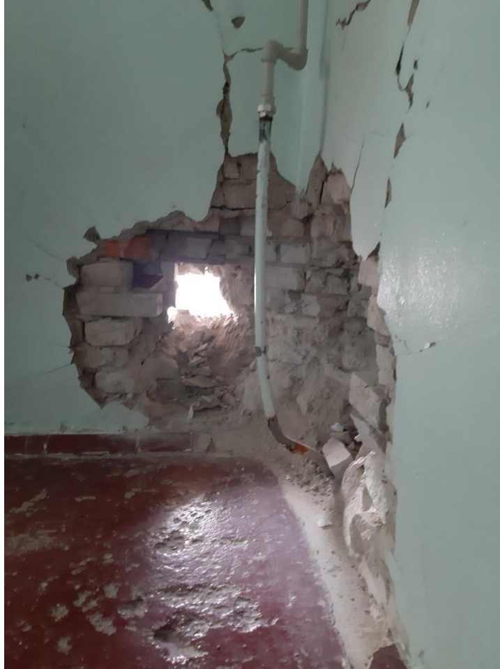
Pic. 4. Damage to the Trostyanets City Hospital after the first attack on March 18, 2022. Captured by UHC with the eyeWitness to Atrocities app. Item ID 133765. See Annex I.
