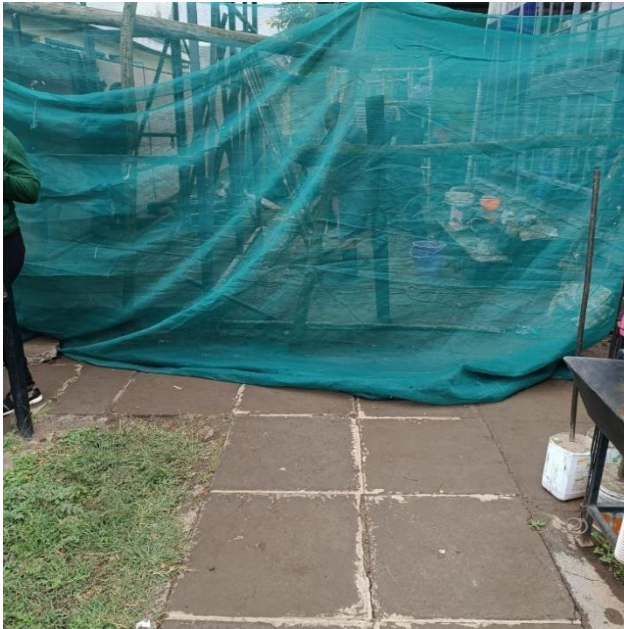
“Here there’s a structure being built and beside it is where the counseling session happens.”
