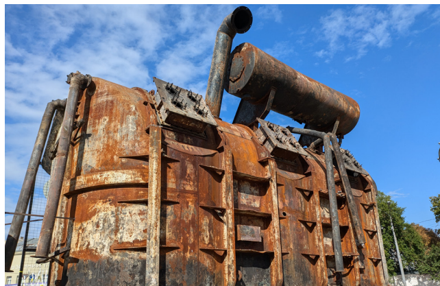
A destroyed power transformer from Burshtynska thermal power plant displayed on a square in Kyiv, Ukraine no longer produces such transformers making them difficult to replace. Photo captured by Physicians for Human Rights in September 2024.
